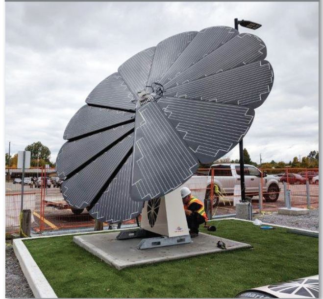
The solar panel array at the Community Energy Park.
